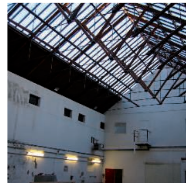
Interior of Earlsfort Terrace Real Tennis court, showing glass roof and full-height partition.
